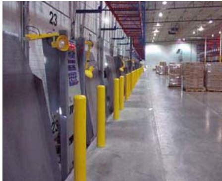
Dock Levelers, M&M Mars Warehouse, Manteno, IL
